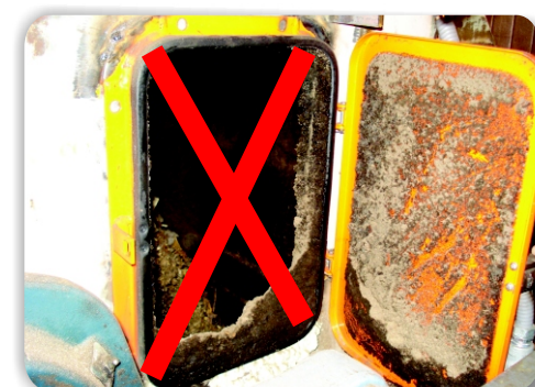
Current inspection door allows for unsafe access to running equipment.
