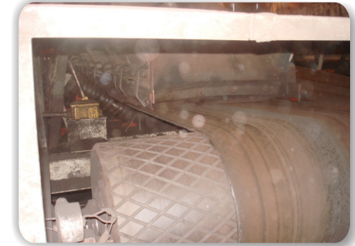
Severe side travel to the right hand side of the tail pulley, causing material spillage and conveyor belt damage.
