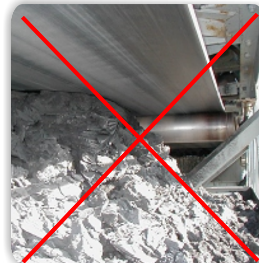
Carry-back accumulations on the return side of the conveyor belt.
