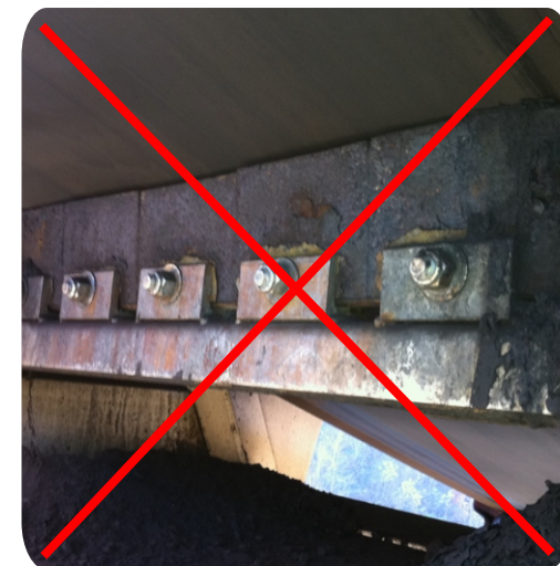
The previous cleaner removed was not tensioned and maintained. The tensioner locked up and seized.
