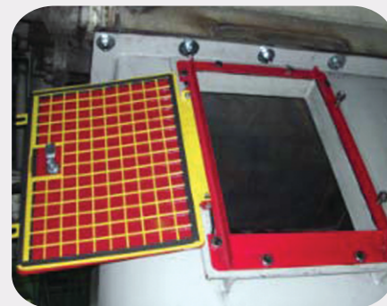
Door opened. Safety screen opened.
